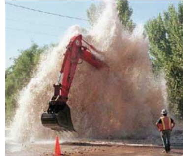
Unexpected Water Main Break
